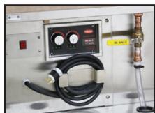
Control Panel, Well Drain
