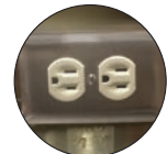
15A - 120V Duplex Receptacle Hidden Beneath Blender Shelf
